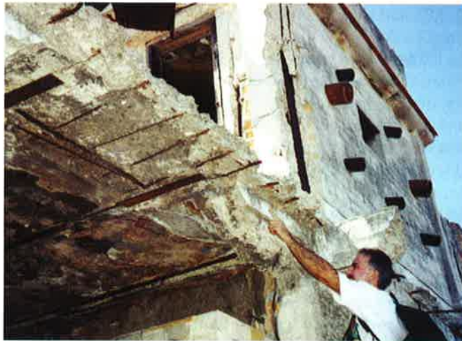
Fig. 1: Corrosion-induced damage in a concrete structure
