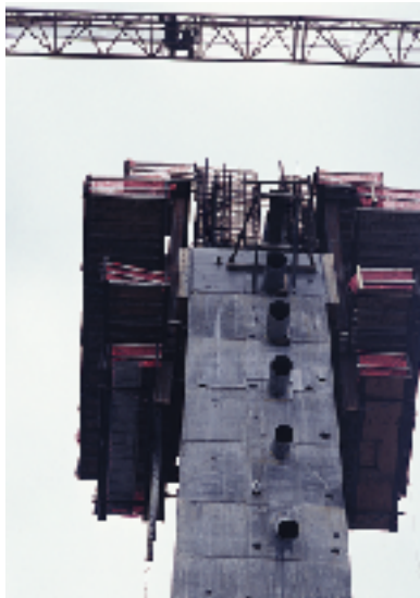
Favorable experience with high-strength concrete prompted Washington DOT engineers to specify 7,000 psi compressive strength mixes for the cable-stay bearing piers of Tacoma's Theo Foss Waterway Bridge.
