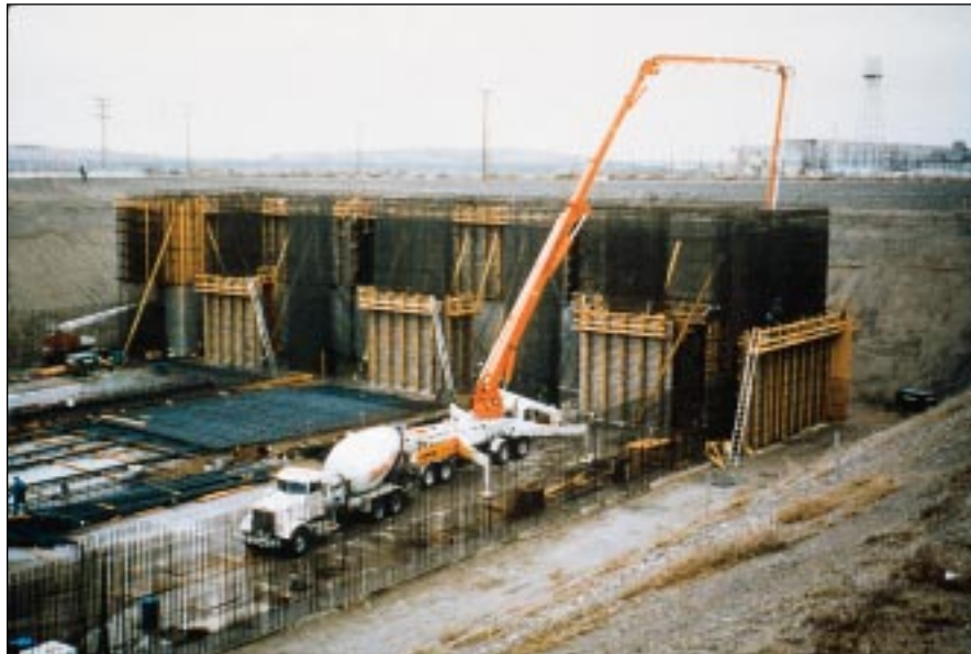
Workability was a major concern because the contractor had to place high-early strength concrete in heavily reinforced walls and slabs by pumping, chutes or buckets.
