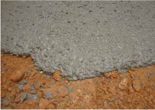
Fig. 2: The SCC mixture exhibited no segregation or bleeding, even after a high-energy drop chute placement in the 70 m (230 ft) deep shaft
